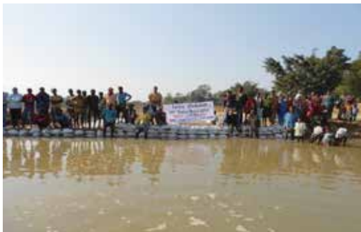
Fig. 4 Sand bank check dam at Jharkhand
