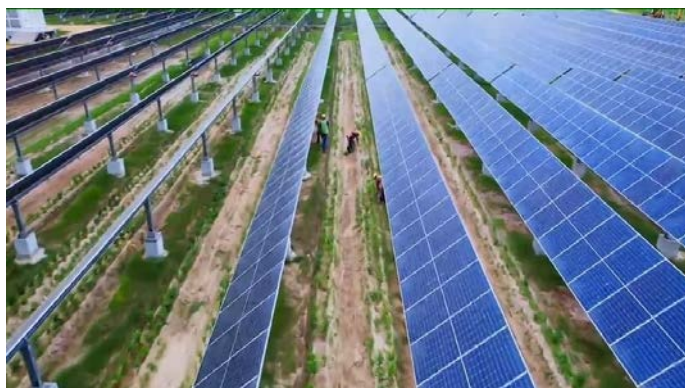
Fig. 40 Sri Lanka's first-ever solar power plant - Vavunathivu
